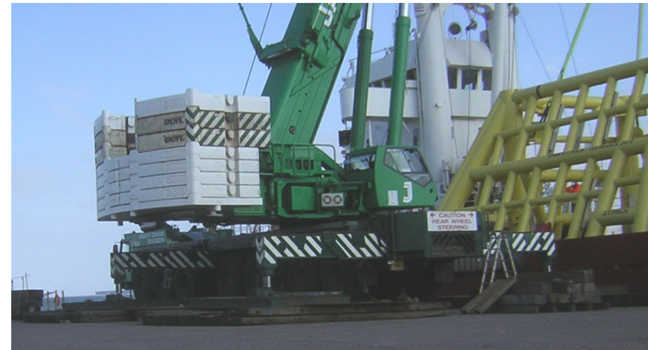
fig. 05/ a layered load spreading arrangement underneath crane outriggers, required to meet allowable ground loading at the port.
